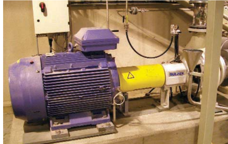
White Liquor Pump showing motor and coupling guard.
