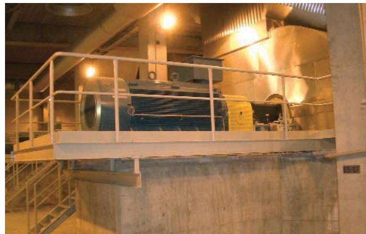
Access platform for Exhaust Gas Fan #3.
