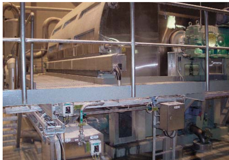
The rotary filter. Accelerometers were mounted on the filter bearings and the gearbox (green, upper right); however, the problem was traced to an unmonitored mixer underneath the filter (concealed in lower left corner of photo).
